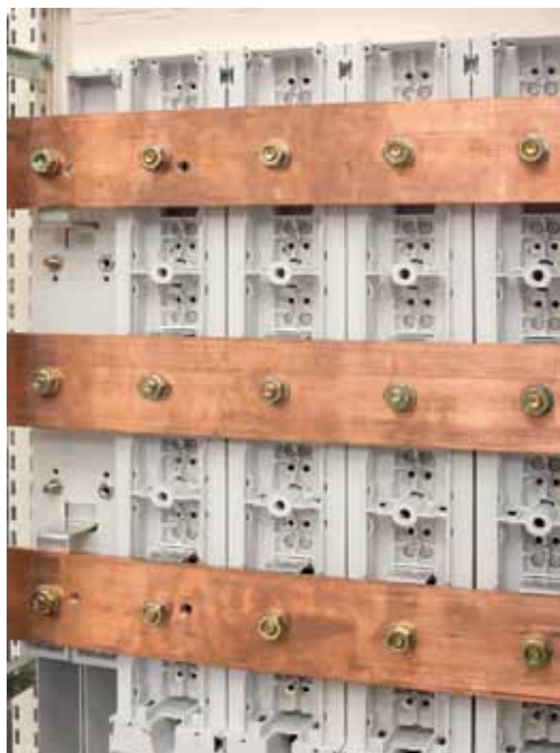
ISFL250 (direct connection on 185 mm² busbar).
